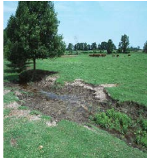
Eroded stream due to unlimited access Photo courtesy of USDA NRCS
